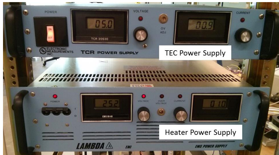
Figure 20. Test Stand Power Supplies
